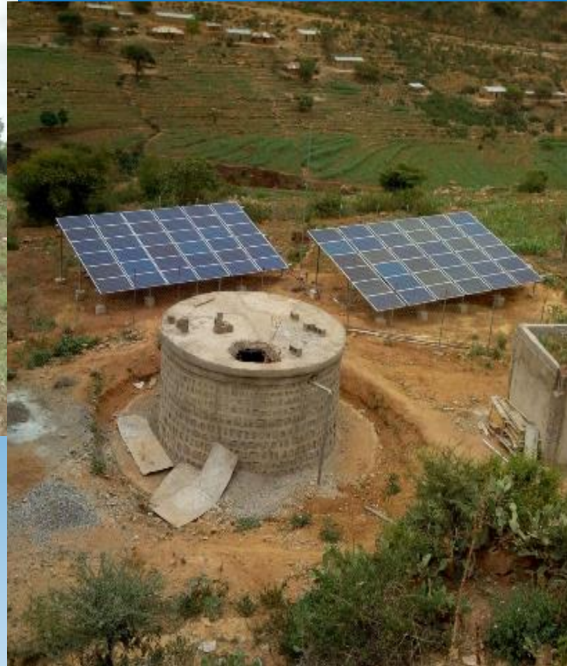
Dire Dawa Village water supply One Borehole (200m 3 /day, 18.5kw) and 3Boosters
