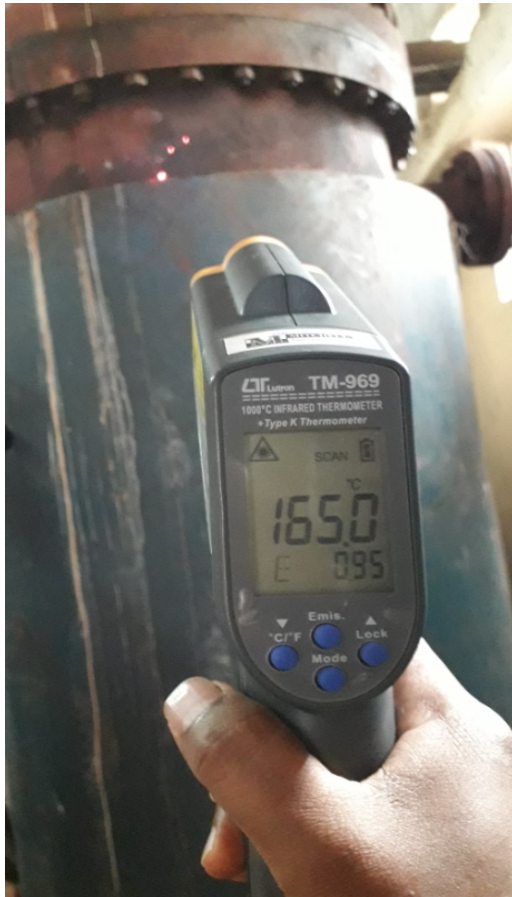
Bare Boiler Surface Temperature
