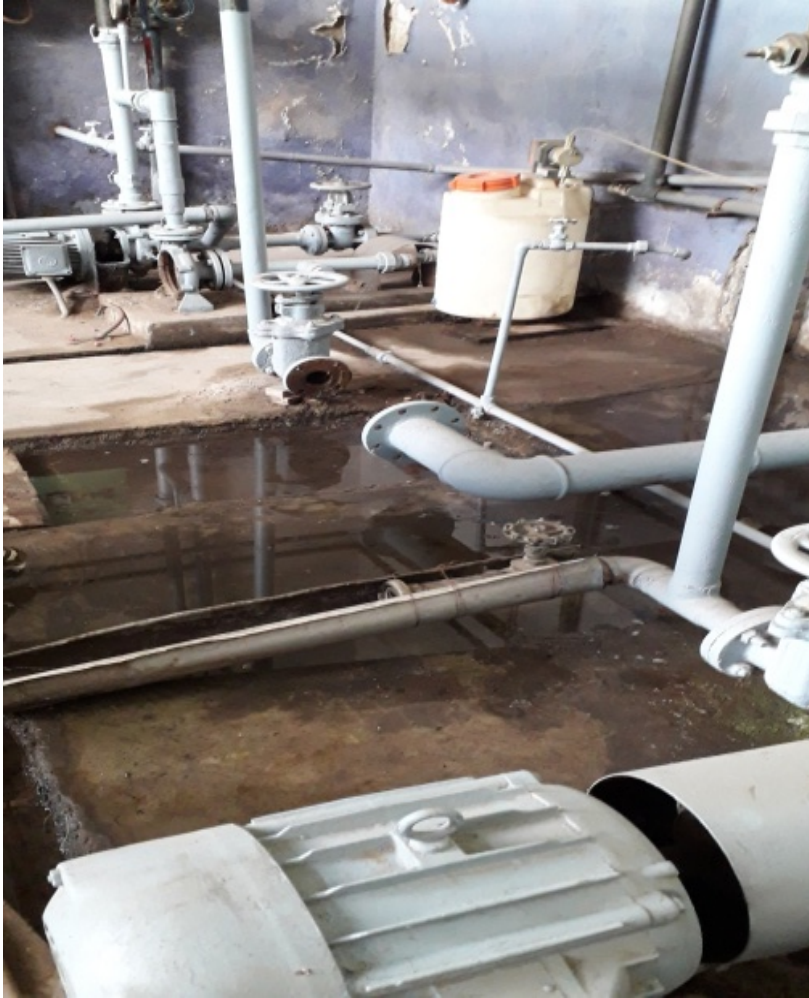
Water leakages (pumping station)
