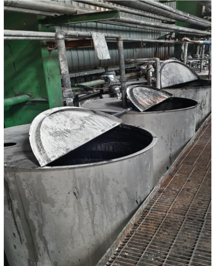
Chemical mixing and transferring
